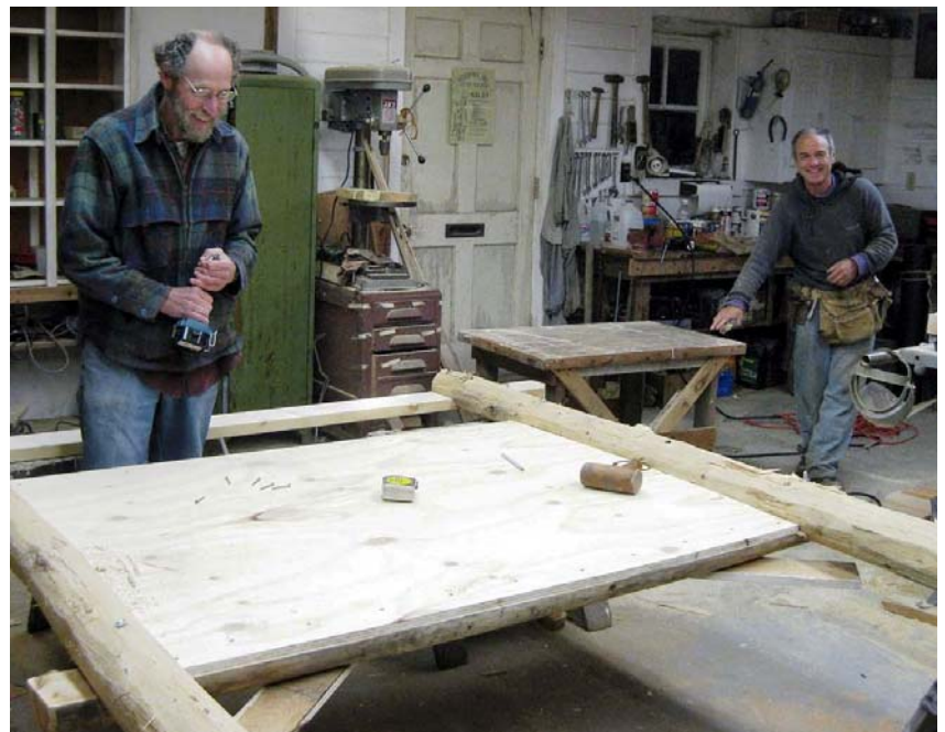
Above: Kiosk construction with smiles! We thank BRCA board members, David Axelman (left) and Roy Bouchard (right), for their time and effort.
