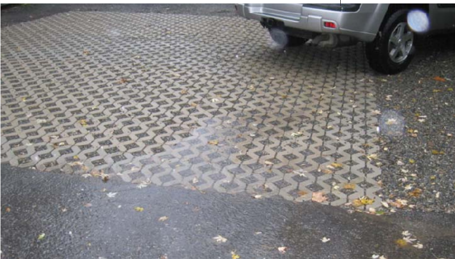
Below: Runoff infiltrating into pervious pavers at Day’s Store.
