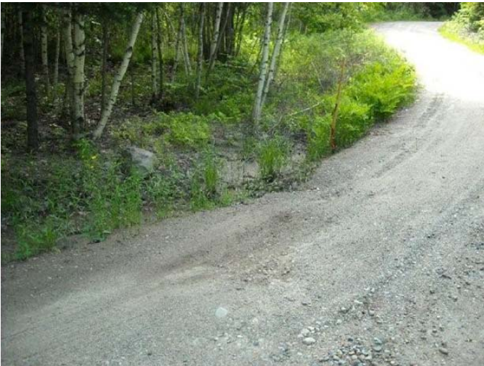
Before: Eroding road surface and totally plugged culvert at Lakewood Estates.
