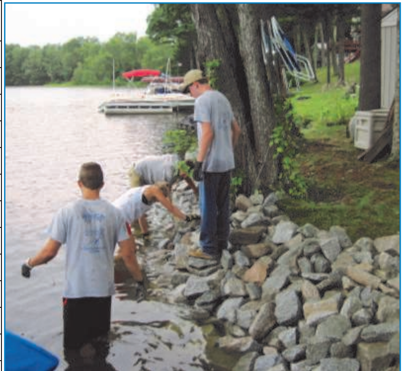
Photo: Conservation Corps crew members installing a riprap project to protect Messalonskee Lake from erosion and phosphorus that is deteriorating water quality.
